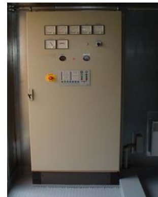
Generator regulation and distribution
