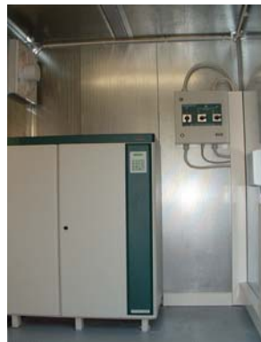
UPS-System 40kW with ventilation System and / or Air conditioning
